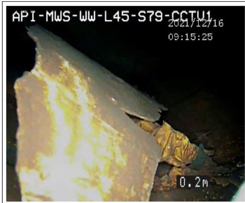
Main at 0.2m flaked lining identified
