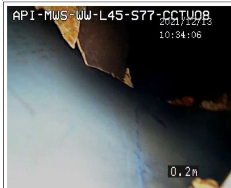
Beginning of survey POI flaked PU lining identified
