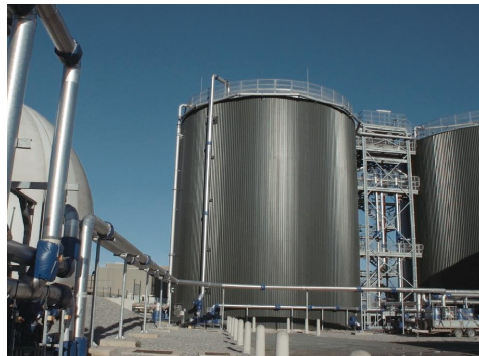
Figure 98 : Five Fords energy park. © Welsh Water
