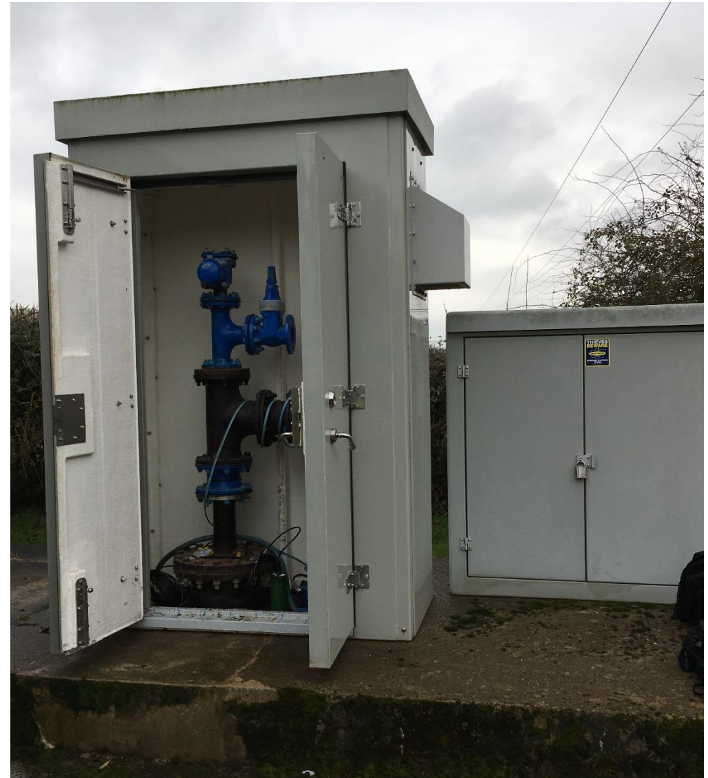
Figure 53 : A small Welsh Water UV treatment plant in Herefordshire. © Arup
