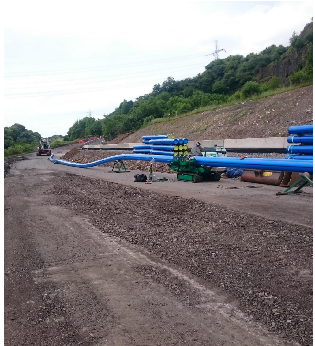
Figure 49 : Water supply pipes on the A465. © Arup
