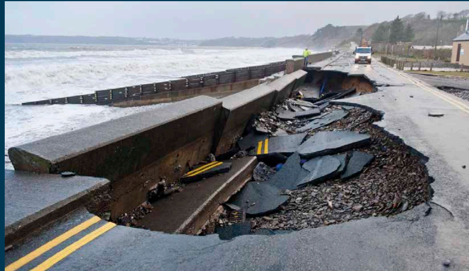
Amroth, Pembrokeshire — Despite the water main being washed away by the stormy sea in January 2014, we restored water supplies to the local community within around 5 hours.
