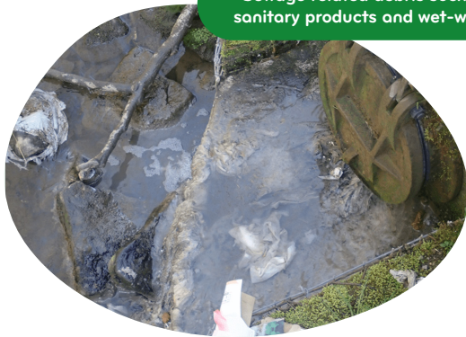
Sewage related debris such as sanitary products and wet-wipes
