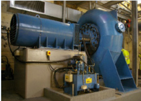
Hydro turbine at Elan valley.
