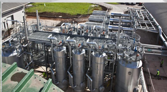
Advanced Digestion Installation at Cardiff Wastewater Treatment Works
