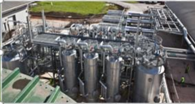
Advanced Digestion Installation at Cardiff Wastewater Treatment Works
