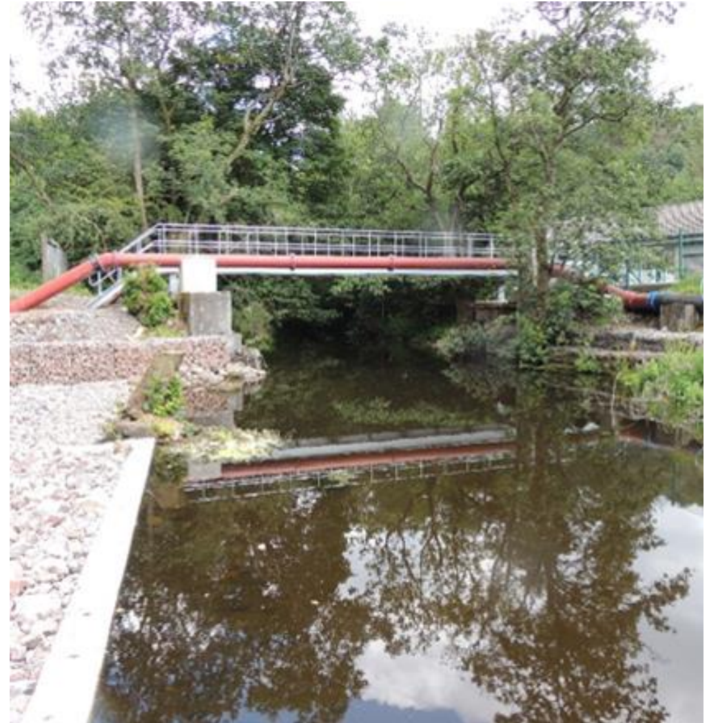
Figure 54: Raised pipe bridge at Pontsticill. © Welsh Water
