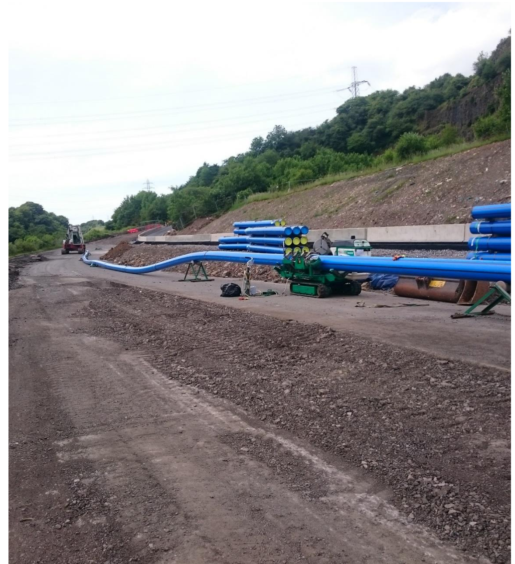
Figure 49 : Water supply pipes on the A465. © Arup
