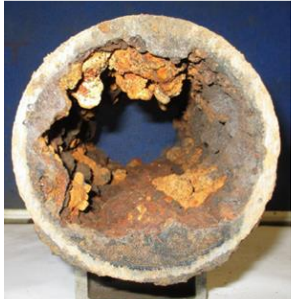
Figure 58 : Iron pipe corrosion. © Welsh Water
