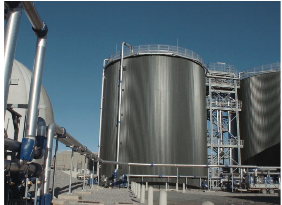
Figure 98 : Five Fords energy park. © Welsh Water
