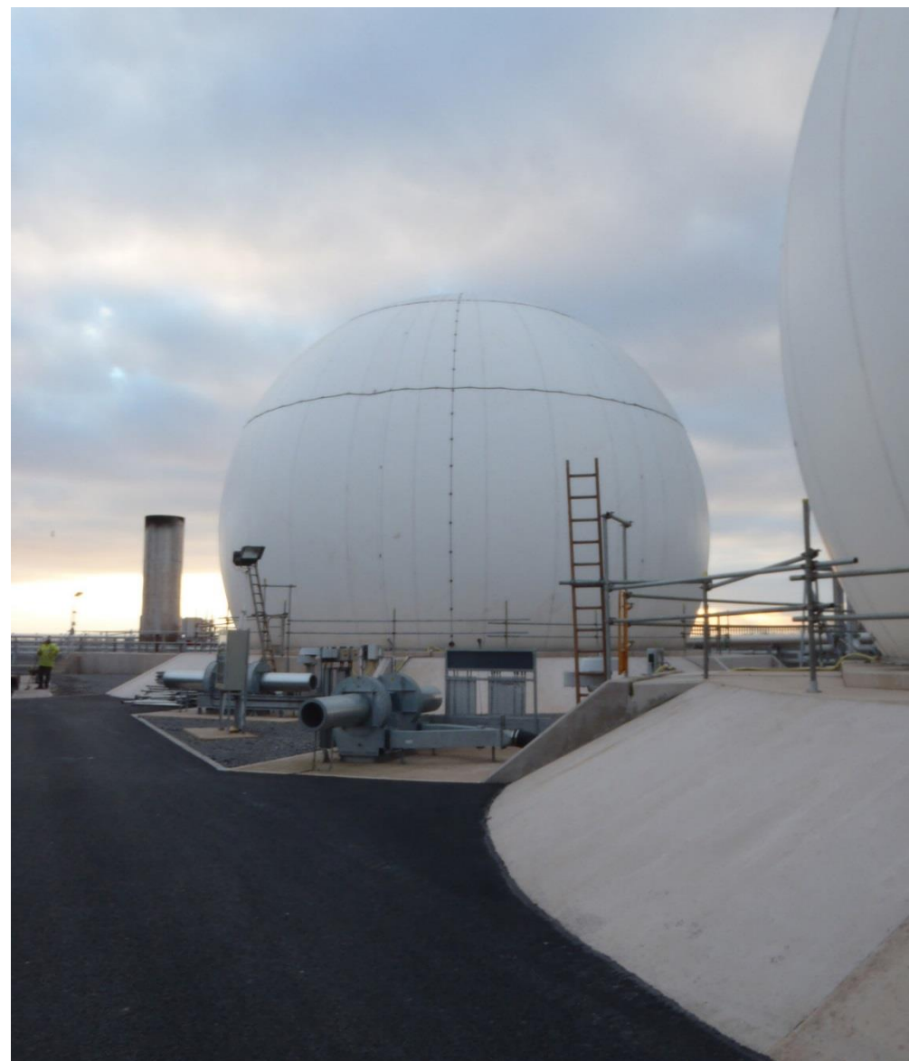
Figure 11 : Cardiff wastewater treatment works advanced digestion facility. © Arup
