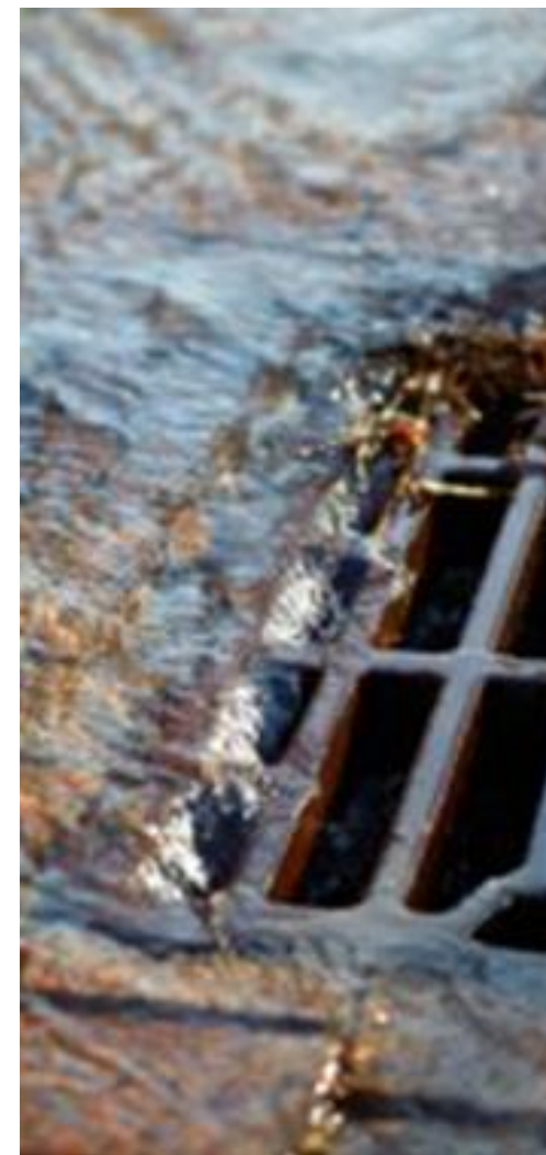
Figure 87 : Drainage © Welsh Water
