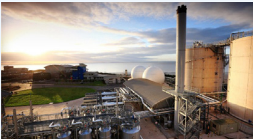
Anaerobic digestion and thermal hydrolysis plant at a Waste Water Treatment Works in Cardiff.
