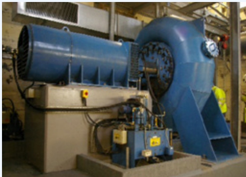
Hydro turbine at Elan valley.
